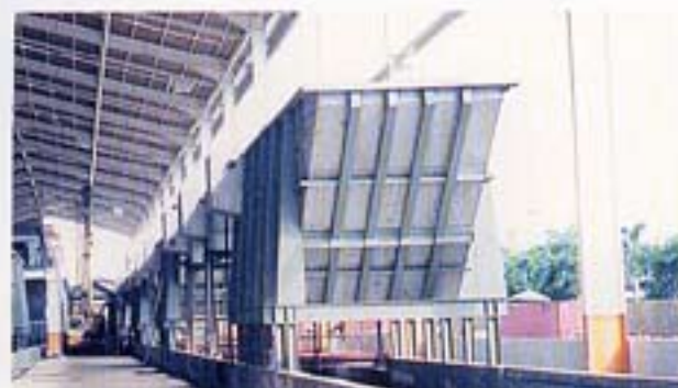
DIP TANK - CAR TOP COAT PLANT
